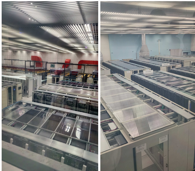
Figure 3-4: Many processing units toiling away in the Data Center
